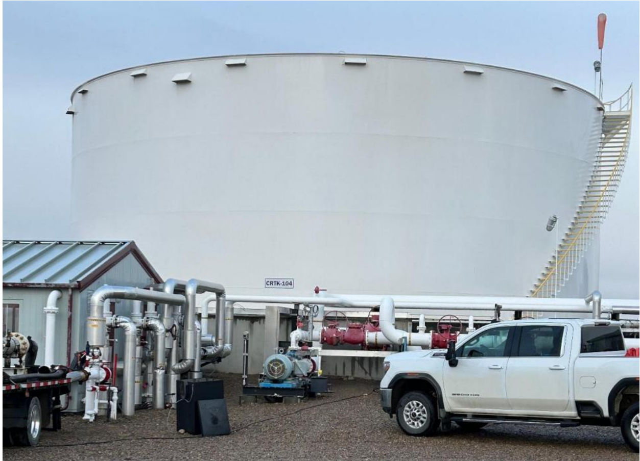
Adjacent Facilities – Tank 104 & Boost Pumps
