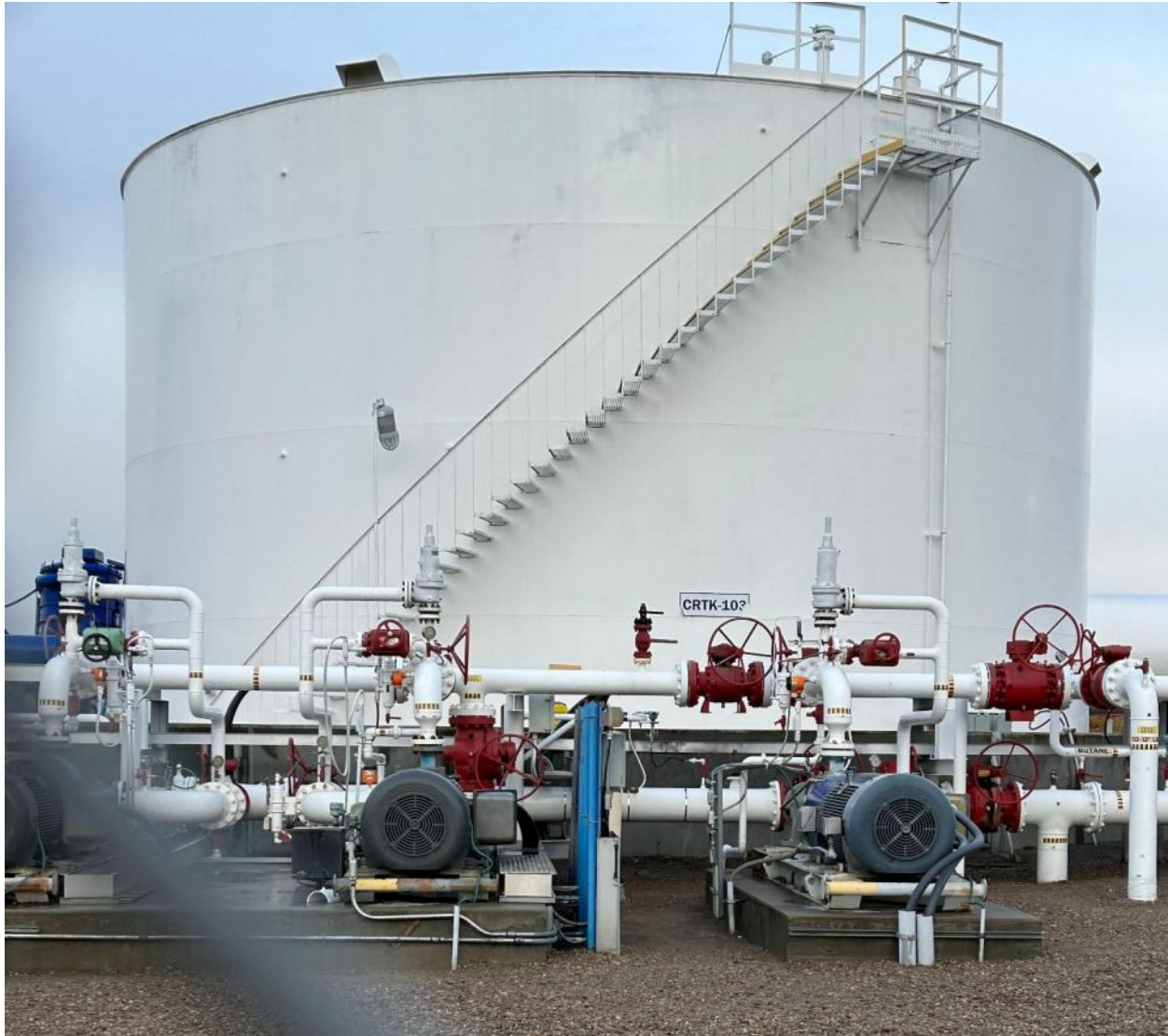
CER Tank 103 & Mainline Pumps
